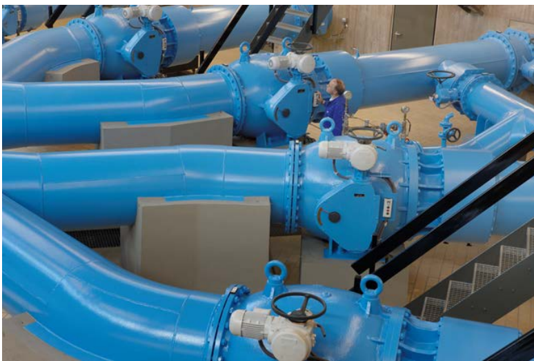
Photo 1: Drinking water distribution pipes in Büttnau
